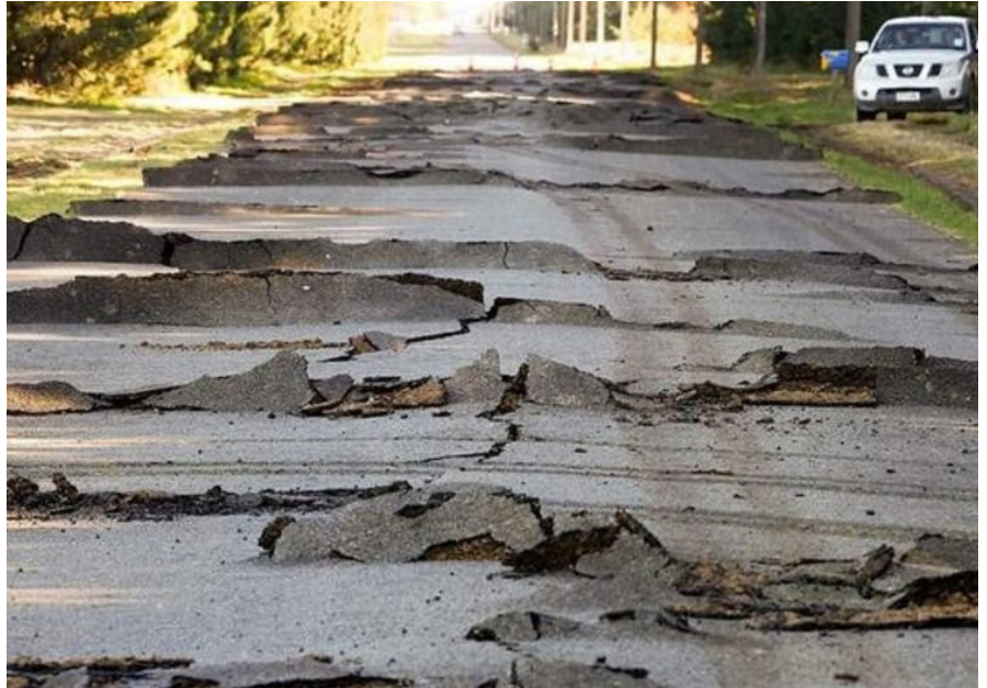
The earthquakes starting in 2010 left Christchurch's infrastructure in ruins
